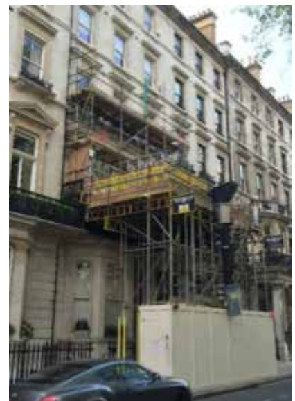
Scaffolding affecting amenity
