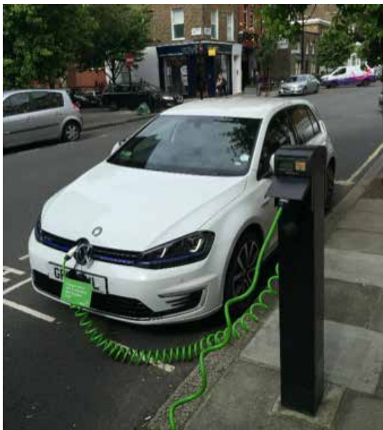
On-street electric charging point
