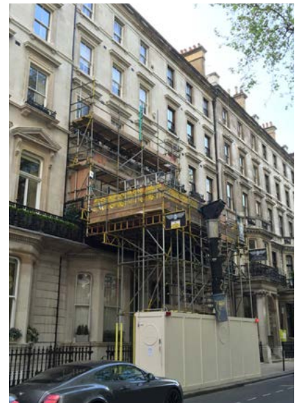
Scaffolding affecting amenity
