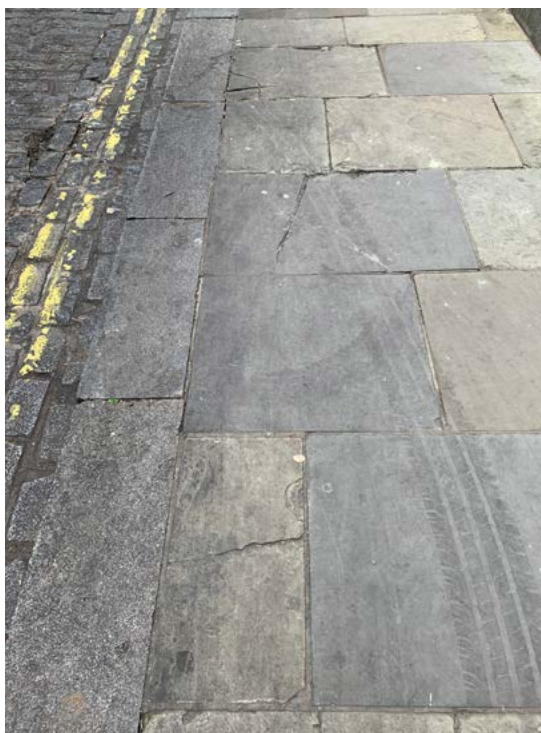
York stone in need of repair in Raphael Street
