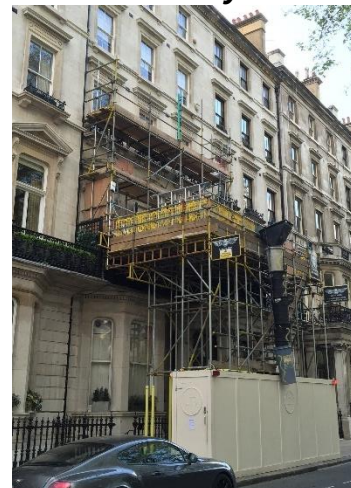
Scaffolding affecting amenity
